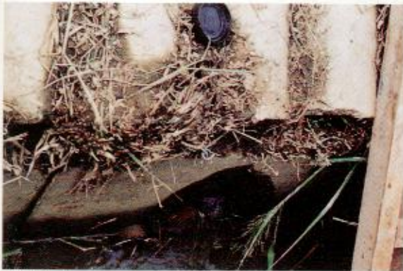
Outlet of subsurface drain pipe
