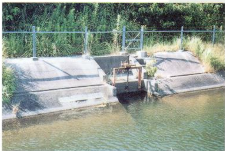
Division or distribution facilities (close-up)
