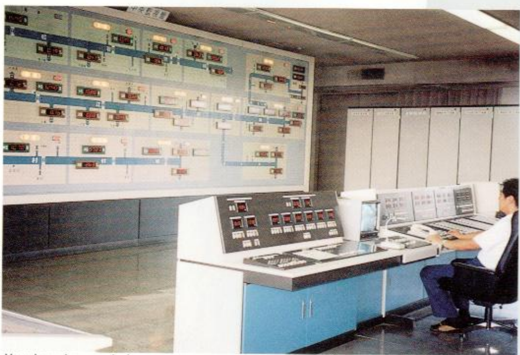
Headquarters control room
