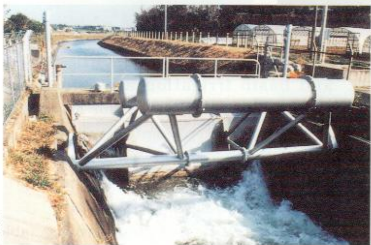
Division or distribution facilities (close-up)
