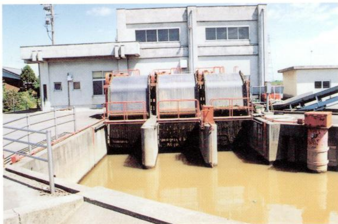
A pump station ( inland side )
